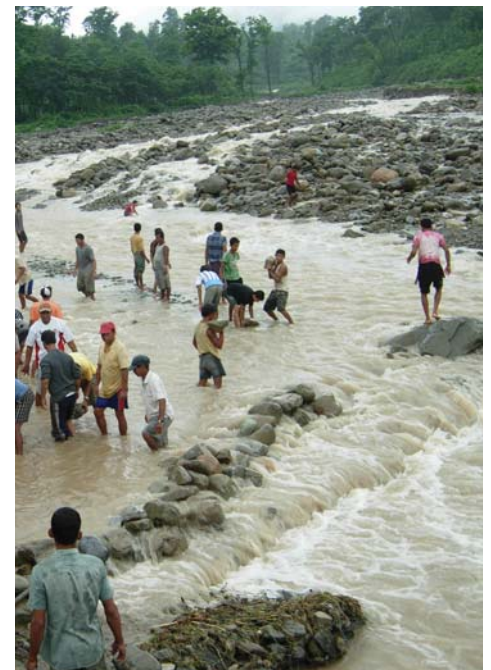
Farmers in Baulaha Khola, Nawalparasi District, Nepal, rebuild flood protection gabions (flood walls), after traditional irrigation channels were flooded.
